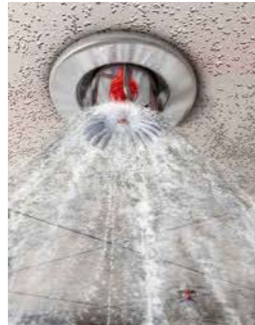
sprinkler fire fighting system
