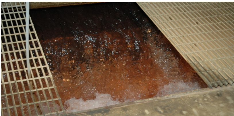
Rapid Mix Tank
