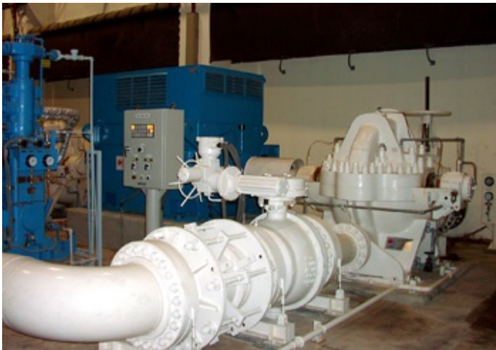
Horizontal Centrifugal Pump
