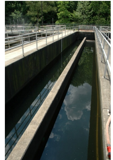
Chlorine Contact Basin106
