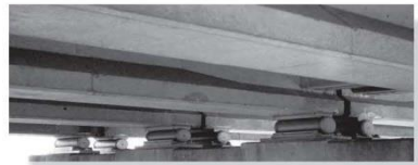
Rollers and associated bearing pads are used to support the prestressed concrete girders of a highway bridge.
