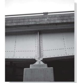
Typical pin used to support the steel girder of a railroad bridge.
