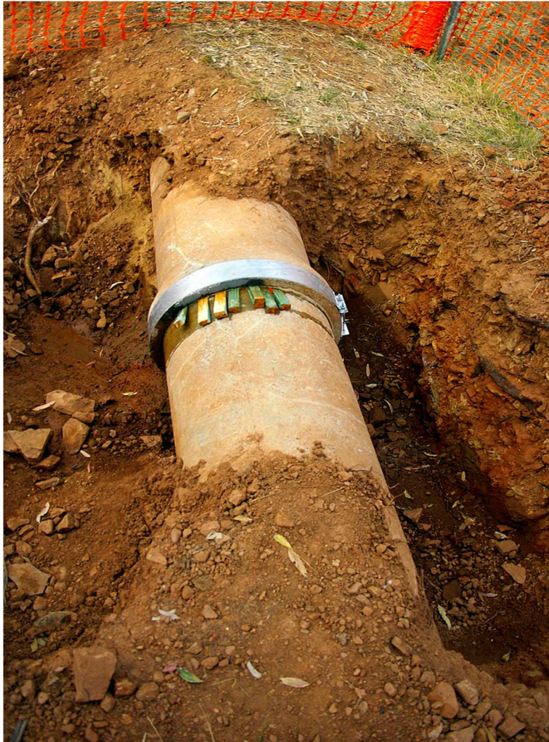
Fig.3 Most (treated) water distribution happens through underground pipes
